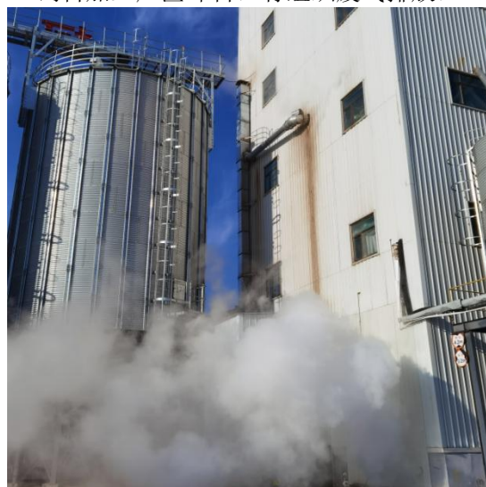
饲料加工车间废气排放口
